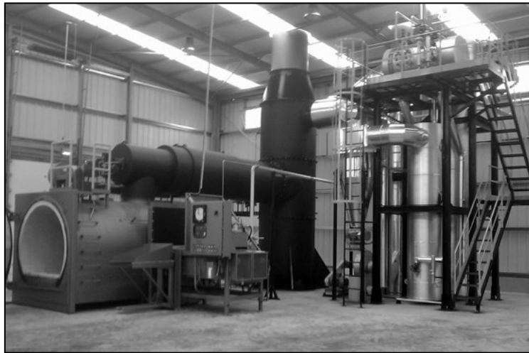
Figure 3: Combustion Chamber at Kualiti Alam.
