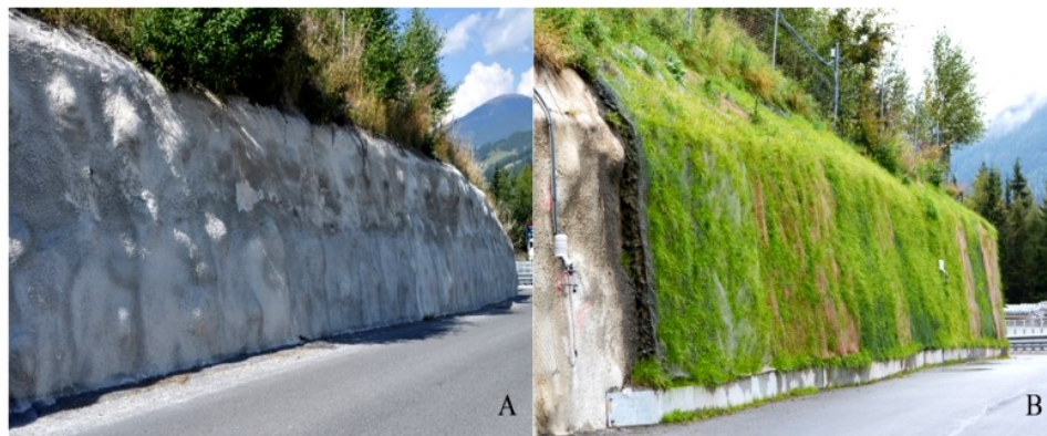
Figure 7: The shotcrete wall along a highway exit (Source: Medl, Mayr, et al., 2017)
