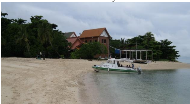
b. Exposed beach and part of the Sabah Parks office. Some damage to the building by strong waves was noticeable.
