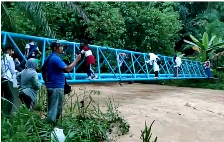
Figure 6. Students crossing water pipe to get to school Source: Anjumin (2022)
