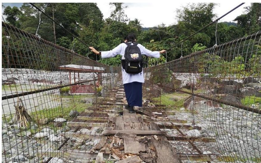
Figure 7. Students crossing dilapidated bridge in Sandakan
